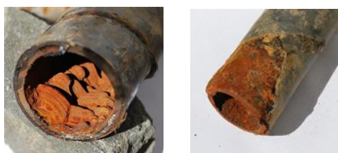
Figure 1. Cold water pipes presenting internal and external corrosion and scaling.
